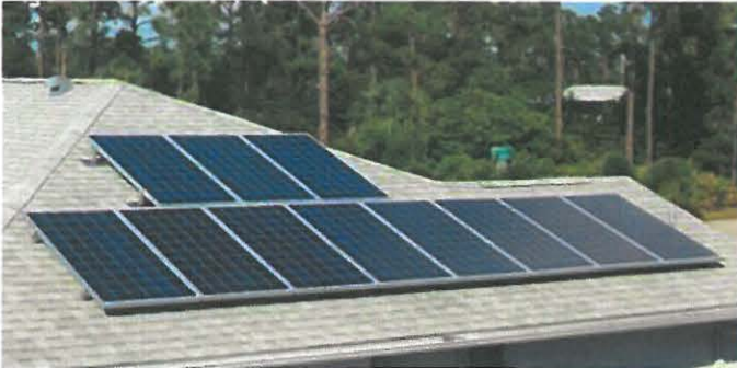
The example shown in the above photo is of a grid-tied solar electric (PV) system. PV module sizes vary and it is difficult to estimate the total system size in watts just by casual observation. This PV array consists of 11 PV modules rated at 230 watts STC each. (Photo Credit – Solar Power Electric™)
